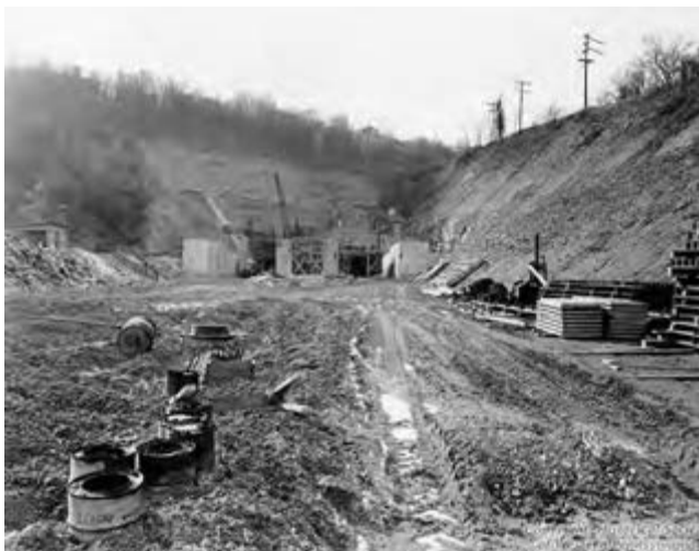
Figure 53. Squirrel Hill Tunnel construction, 1953 (Collier, 2014; taken from Historical Society of Western Pennsylvania).
