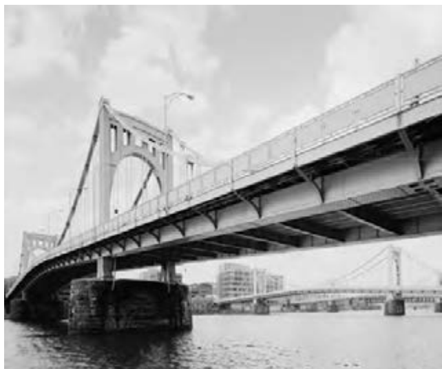
Figure 50. Sixth Street Bridge in downtown Pittsburgh: Historic American Engineering Record collection (Cridlebaugh, 1999).
